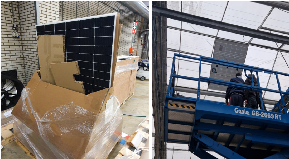
Figure 37: PV panel to be installed (left) and the first PV panel being installed (right)
